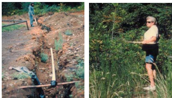
The trench dug through rocky soil is readied for the water line in 1985. June Schuck, clipboard in hand, reviews plans for the water line and irrigation system.
